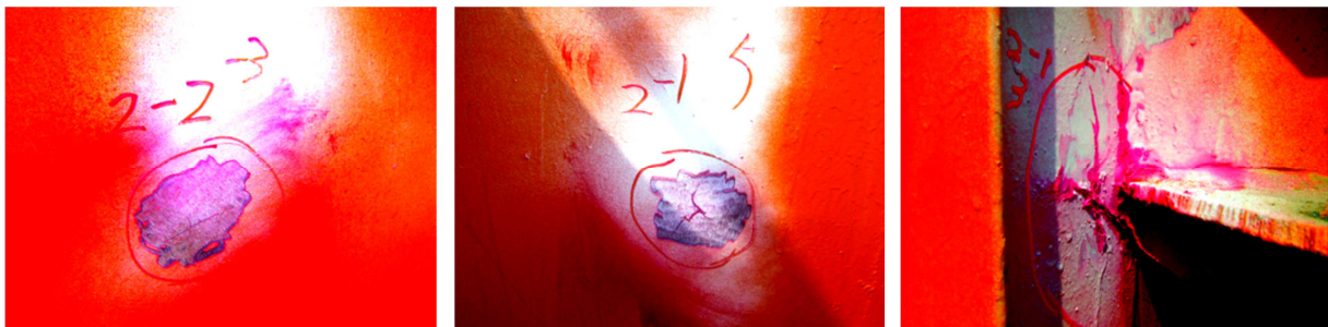
Figure 8. Cracking defects of the main beam of the rotating platform.
